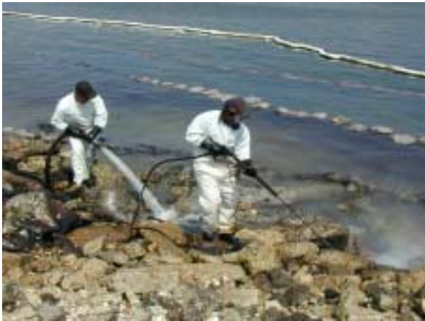
Steam cleaning and cold water flushing of broken concrete rip rap. Sorbent booms and snare catch released oil
