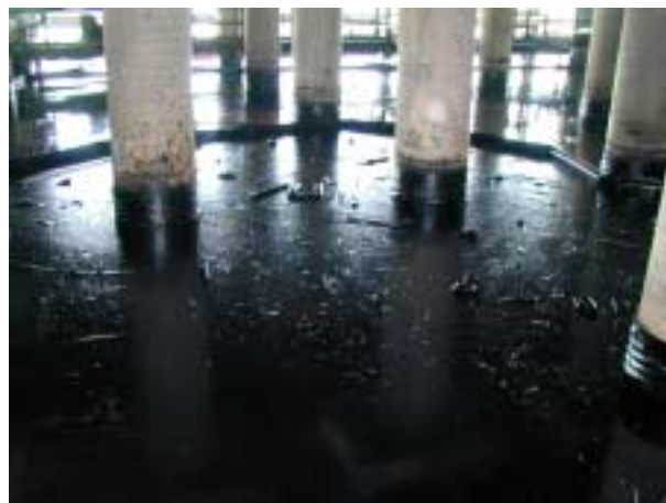
Floating black oil beneath the quay before the "Big Flush"
